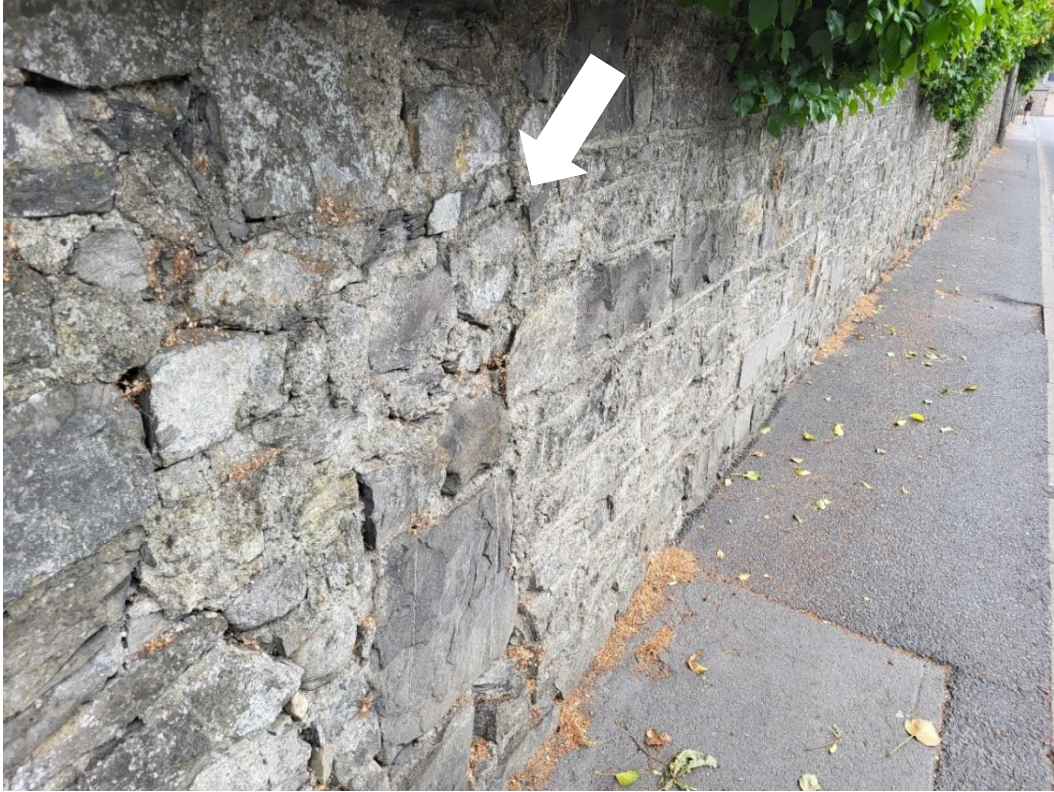
Figure 5 The seams between the original sections of the Demesne boundary wall on either side of the infilled section can clearly be seen on closer inspection. The random rubble masonry of the original boundary on the left, with the neater blockwork of the infill on the right.
