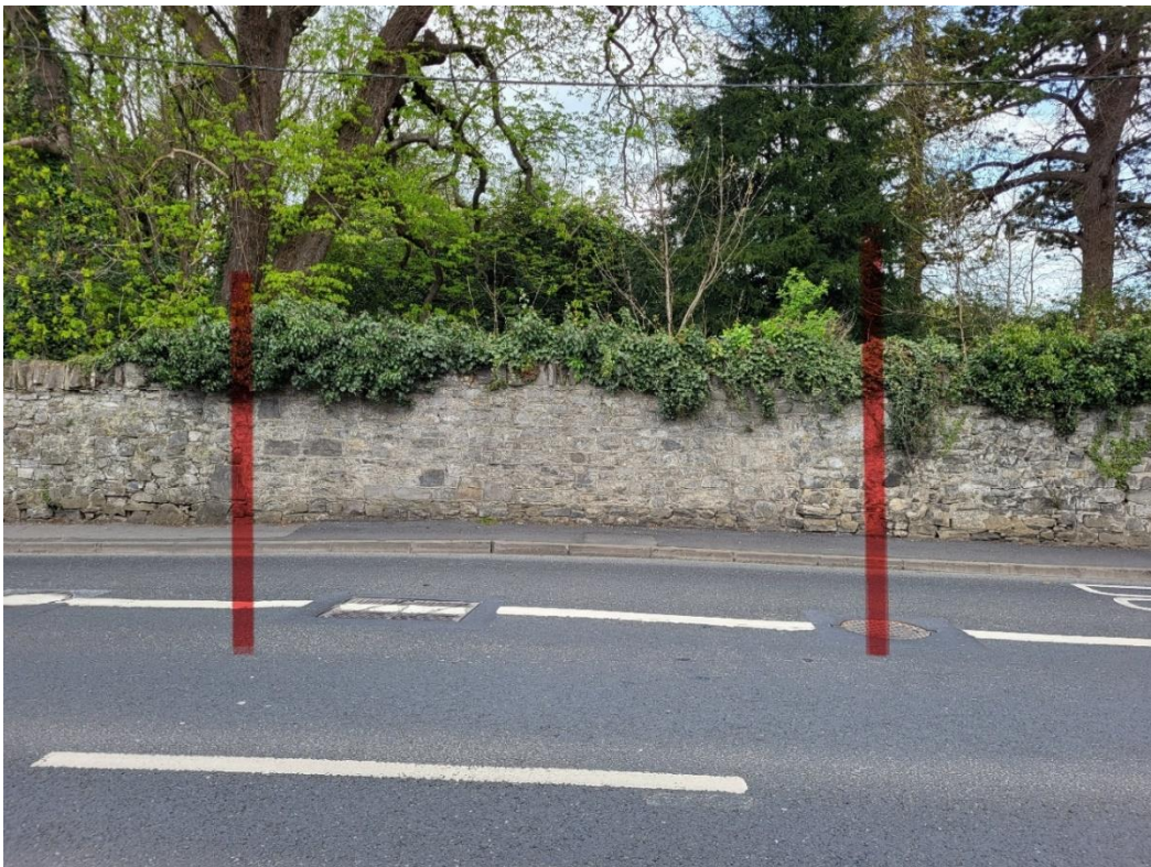
Figure 4 The section of infilled wall that replaced the original bow-fronted projection in the Demesne boundary wall is indicated by the red lines. The composition of the masonry is noticeably different. Without referencing old maps to see that a projection once existed, one would think that the wall was simply repaired.
